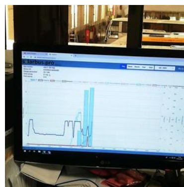
Figure 8: Solarbus.pro monitoring system
